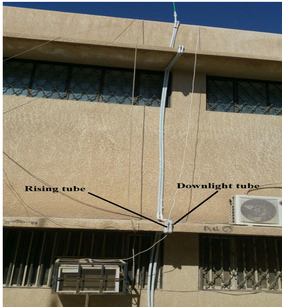
Fig.4.7: shows the supply and return insulation pipes
