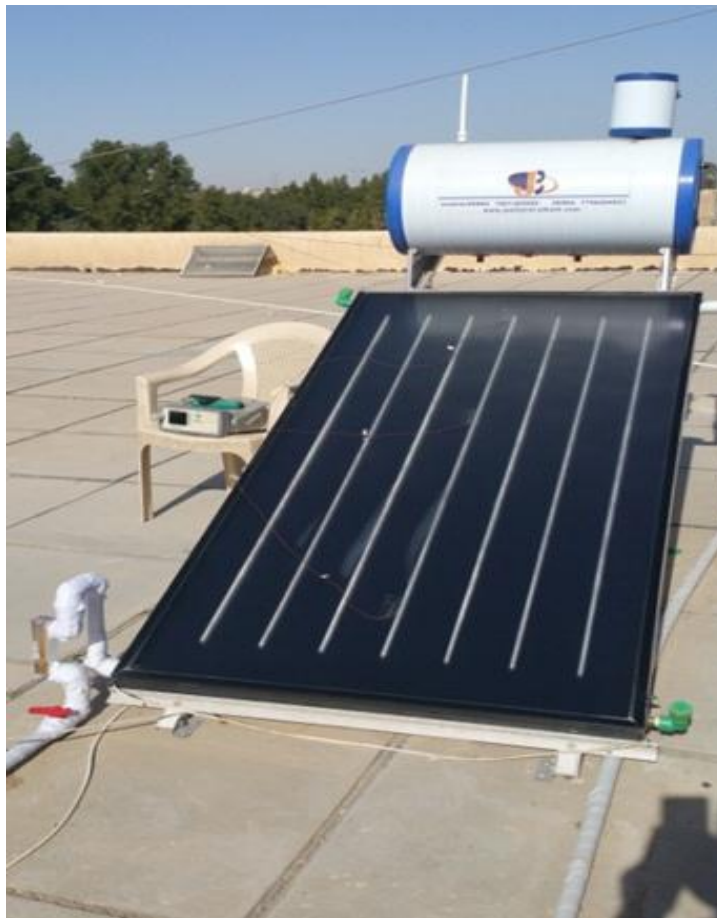
Fig.4.2: Flat plate collector
