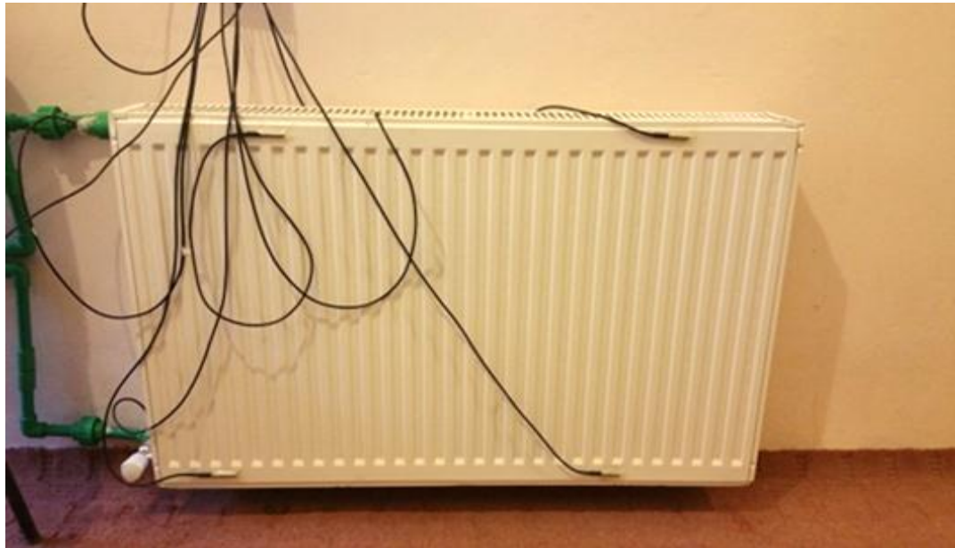
Fig.4.6: The indoor heating radiator
