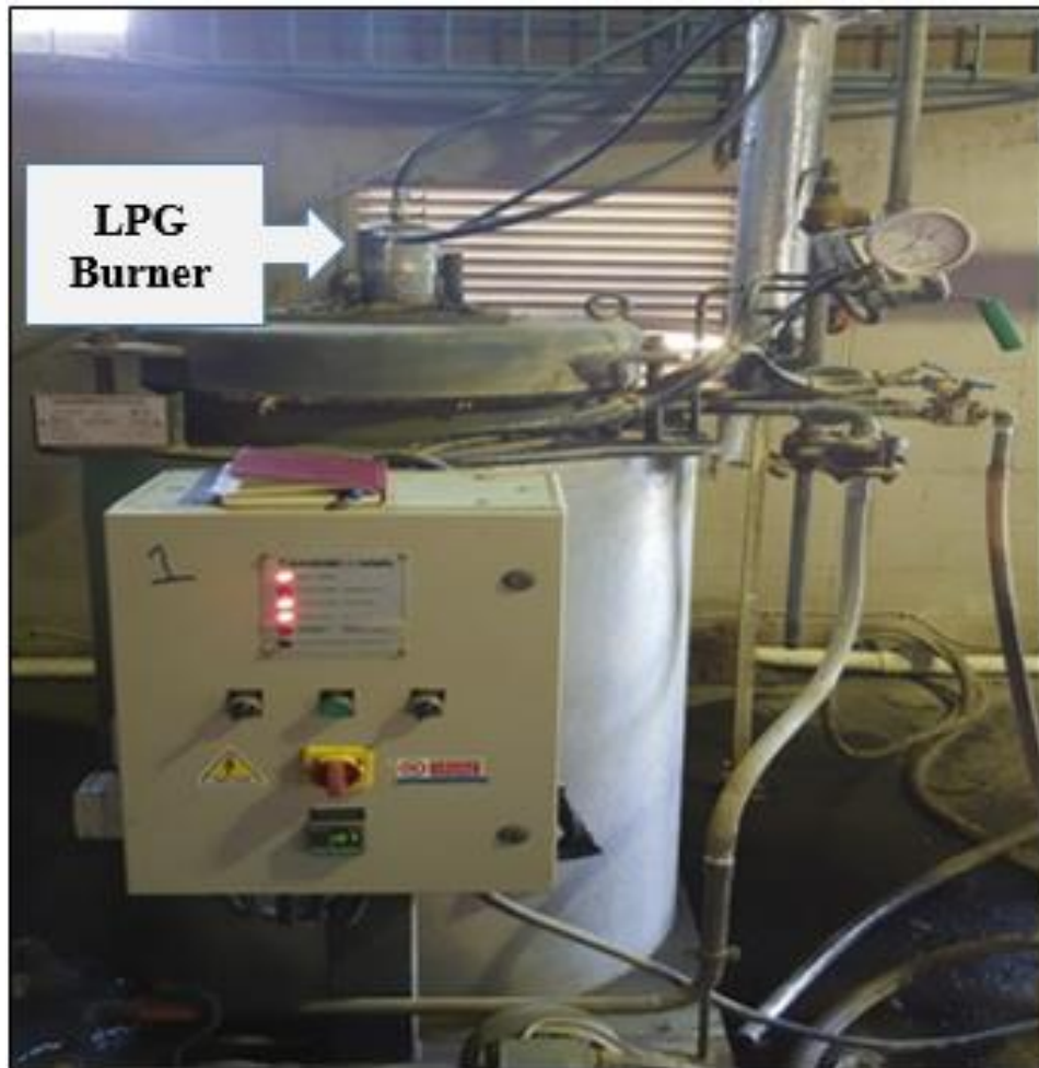
Figure 3.18: General View of LPG Steam Boiler
