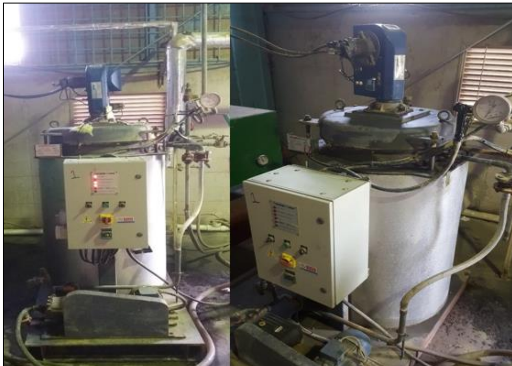
Figure 3.9: Boiler by using Diesel Fuel Burner
