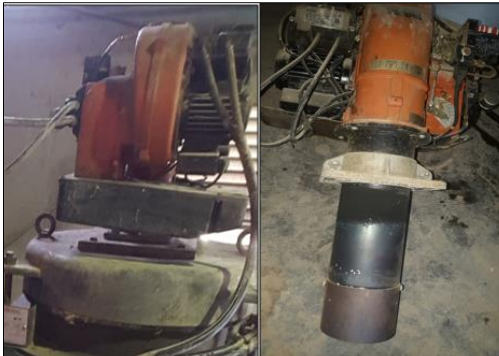
Figure 3.7: Italian Burner Used in the Steam Generation System (Diesel Fuel)
