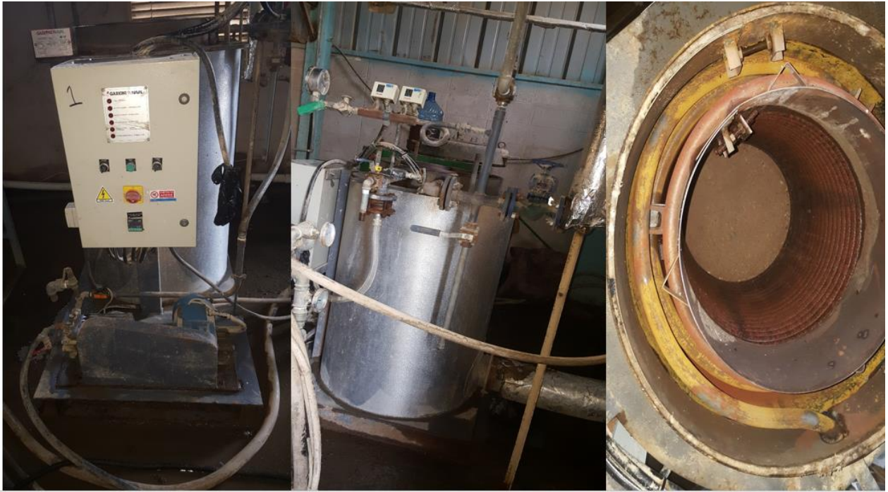
Figure 3.6: Steam Boiler after Rehabilitation
