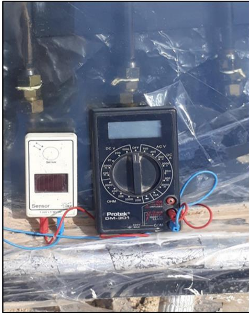
Fig. 4.9: Solar power meter.
