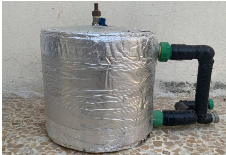
Figure 4.8 cylindrical water tank
