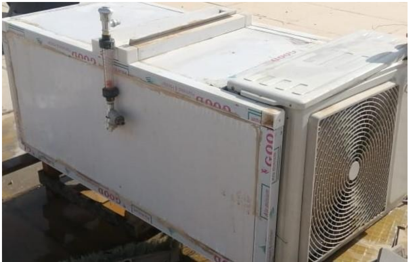
(c) Duct with out door unit
