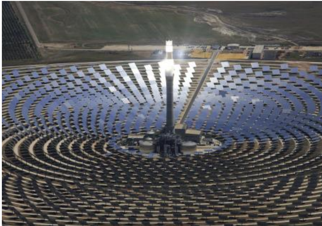
Figure (1.10): Solar tower power generation of Gemasolar plant owned by Torresol Energy, Spain. Picture provided by SENER, Spain, 2018.
