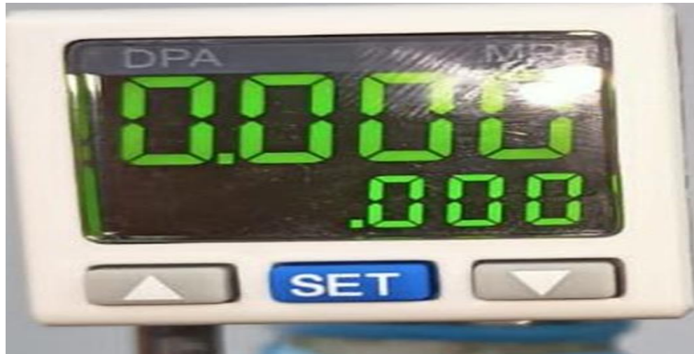
Figure 3.5- Pressure transmitter, DPA-Mpa.
