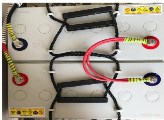
Figure 4.9. Store DC Current (NewMax Batteries)
