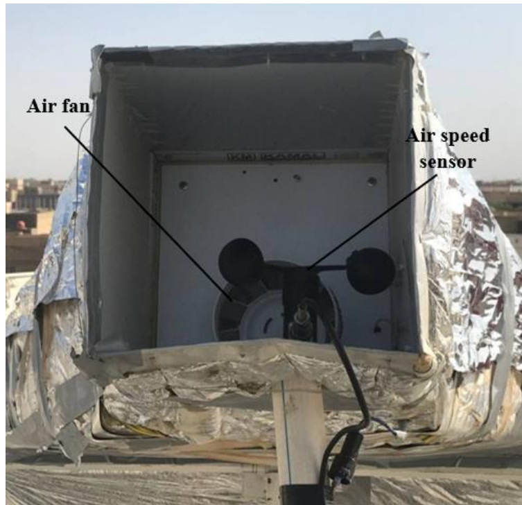
Figure c 3. Air fan and airspeed sensor.
